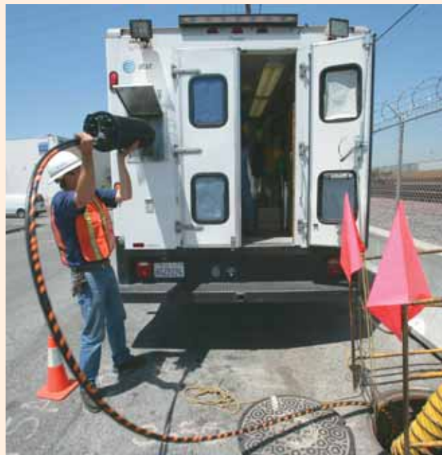
A worker for AT&T prepares to work on a fiber optic installation in Los Angeles. AT&T took over the top spot in the 2008 Top 50 Utility & Telecom Fleets after acquiring BellSouth and Cingular Wireless.
