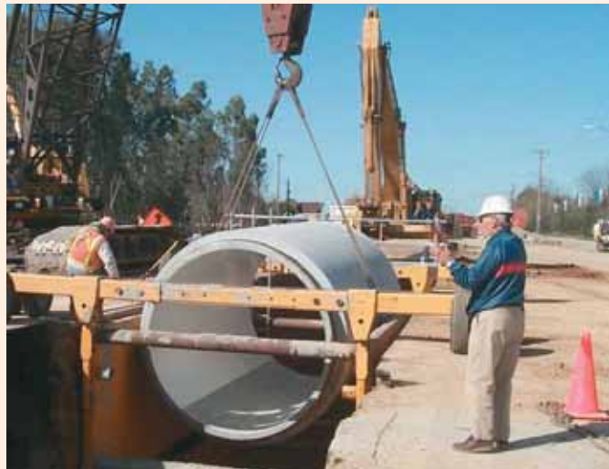
Workers replace pipes in Atlanta as part of the city's water and sewer infrastructure improvements.
